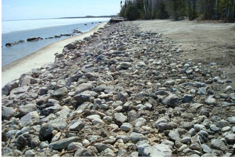
Completed protection barrier in front of lots 5, 6, & 7 Sleepy Hollow, May 2008 (photo taken by complainant)
